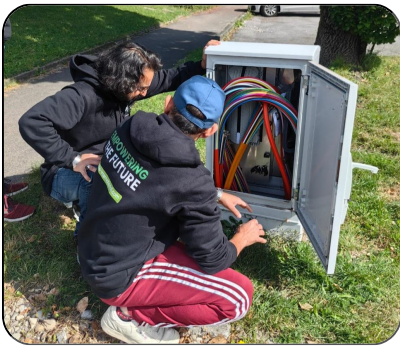
NETS Starts FTTX Deployment in Germany
